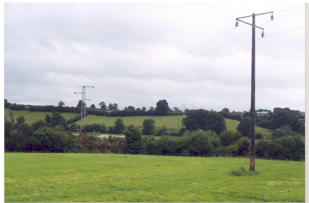
Fig. 4 Siemens 38kV Steel Tower/Wood Pole Line
